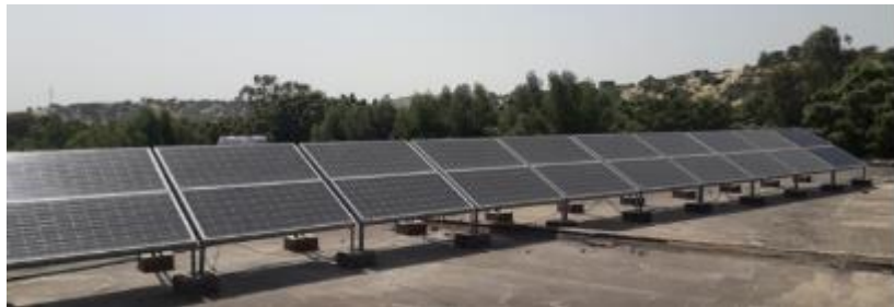
Solar Panels installed at the main campus and some regional campuses
