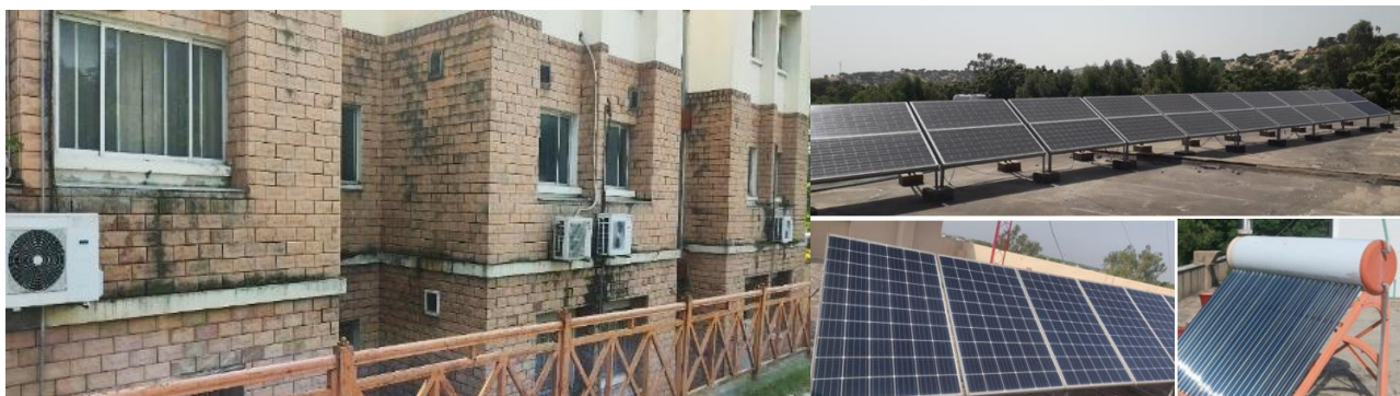
Energy efficient inverters (Combined Cooling Heating and Power Integration Unit) and Solar Panels installed at main campus and some regional campuses
